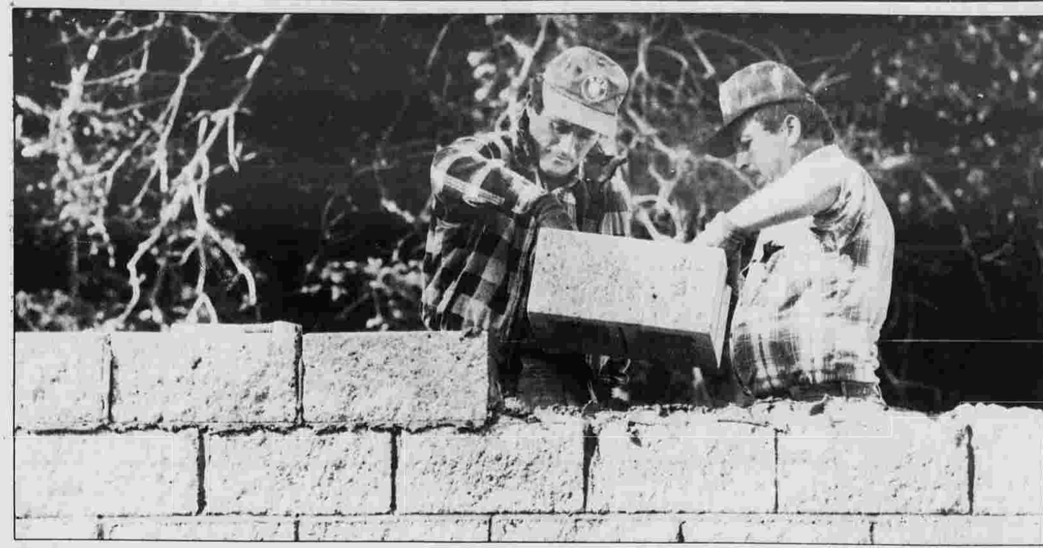
HELPING HANDS — Ted Bineasz, left, and Miroslaw Wondolowski, both of New Britain, work on the new Society for Savings building on Main Street Wednesday. The two are employed by Damiaty Masonry of Cromwell.
